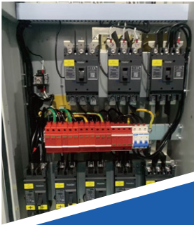
Lightning arrester circuit breaker leakage switch
